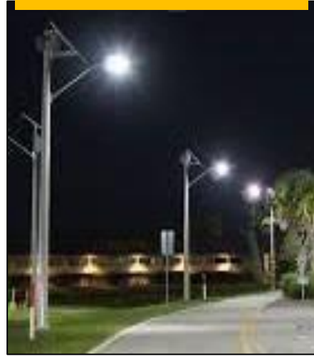
Solar Street Lights: 55 Nos
